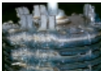
(Contaminated Magnom core after only 6 weeks operation - Bridgnorth Aluminium Hot Rolling Mill Transmission)
